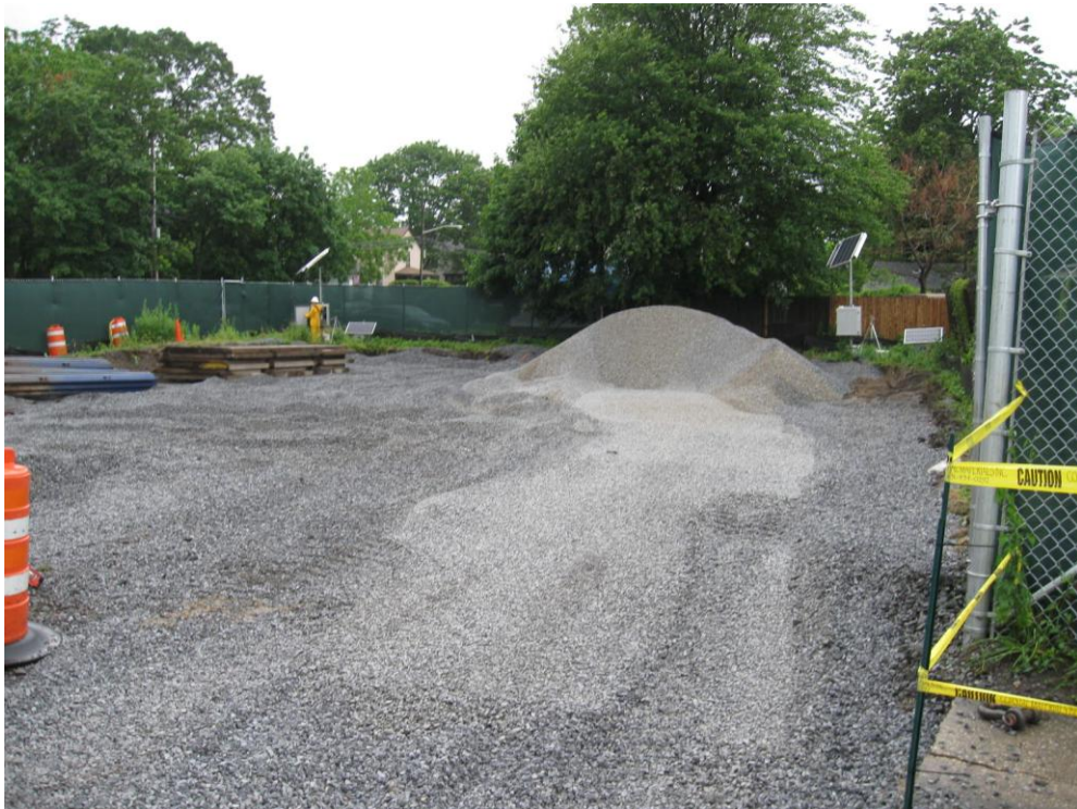
Phase 1 excavation area backfilled with stone to just above the water table.
