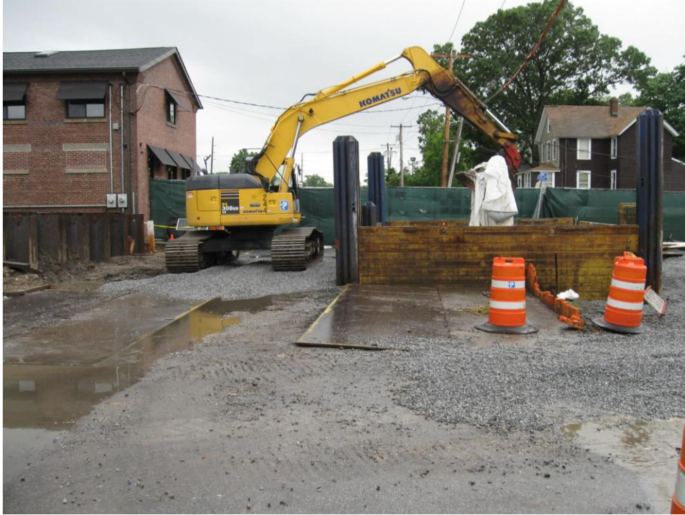
Installation of the first two slide rail boxes in the north side of Oak Street.
