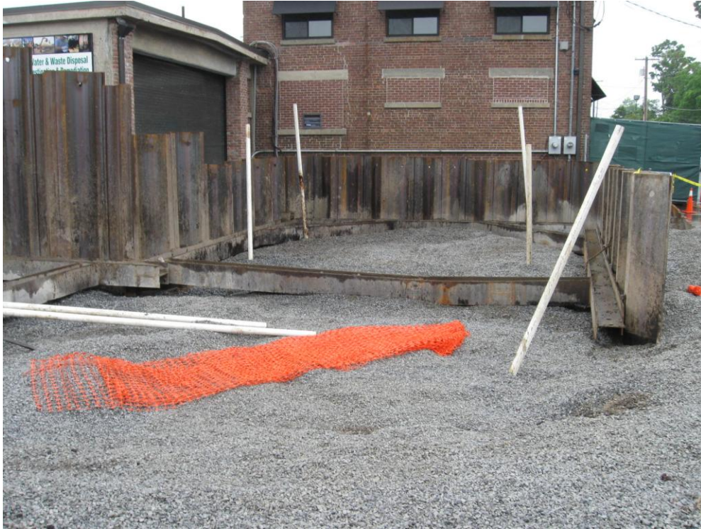
Phase 2B excavation area backfilled with stone to just above the water table.
