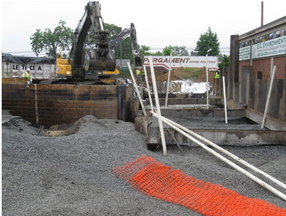
Phase 2B sheet and slide rail excavation east side of 22 Oak Street.
